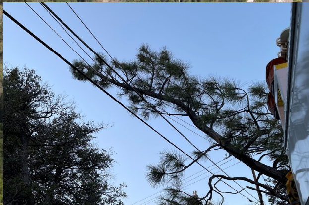
Damage/hazards found after strong winds during PSPS
